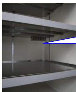
Main sensor E2 in the freezer
